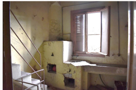
Image-3: The boiler set on terrazzo counter in the washing room.
